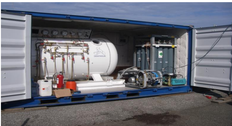
Figure 5. The hyperbaric chamber deployed on site for all the duration of the preparation and of the refloating.
